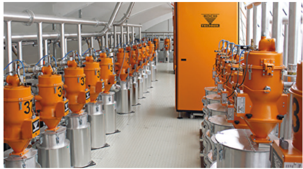
A central granulate dryer system with a total of three CKT type dry air dryers installed at Procter & Gamble Manufacturing GmbH 38 drying containers with a dry air volume of up to 1,600 m 3 /h
